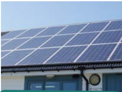
Portland Bill – solar panels above shop and ice cream building by Elliott Brown
